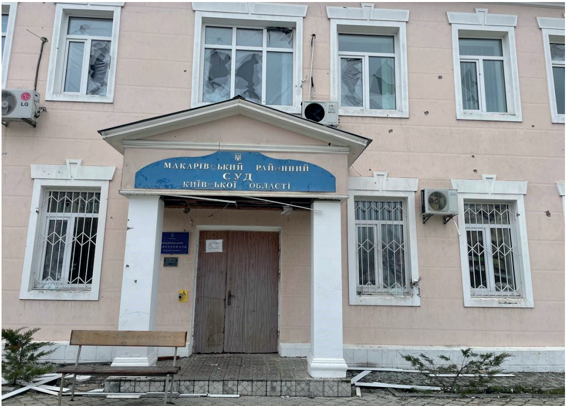
The building of the Makariv District Court of the Kyiv Region after the occupation
